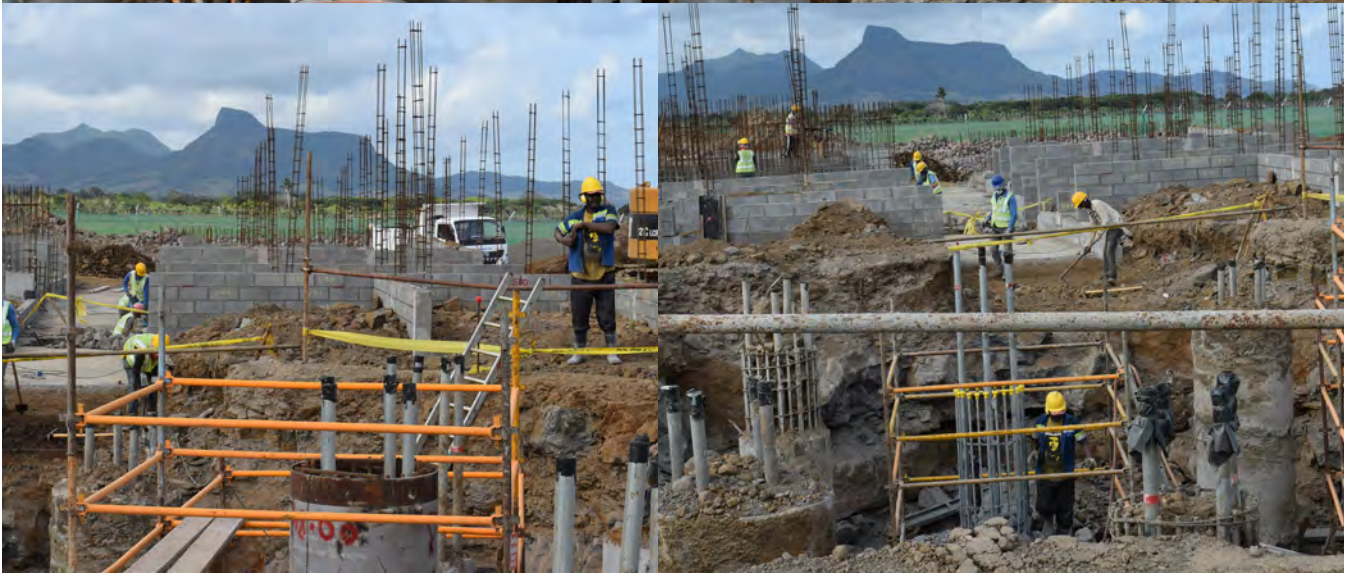
AML - Construction of a new Traffic Control Tower at SSR International Airport
