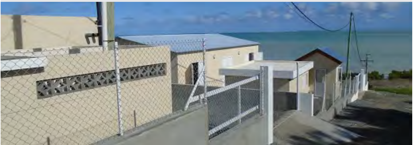
RRA - Supply, Installation, Testing and Commissioning of Reverse Osmosis, Desalination Plants and Equipment at Bay Malgache and Pointe Cotton, Rodrigues
