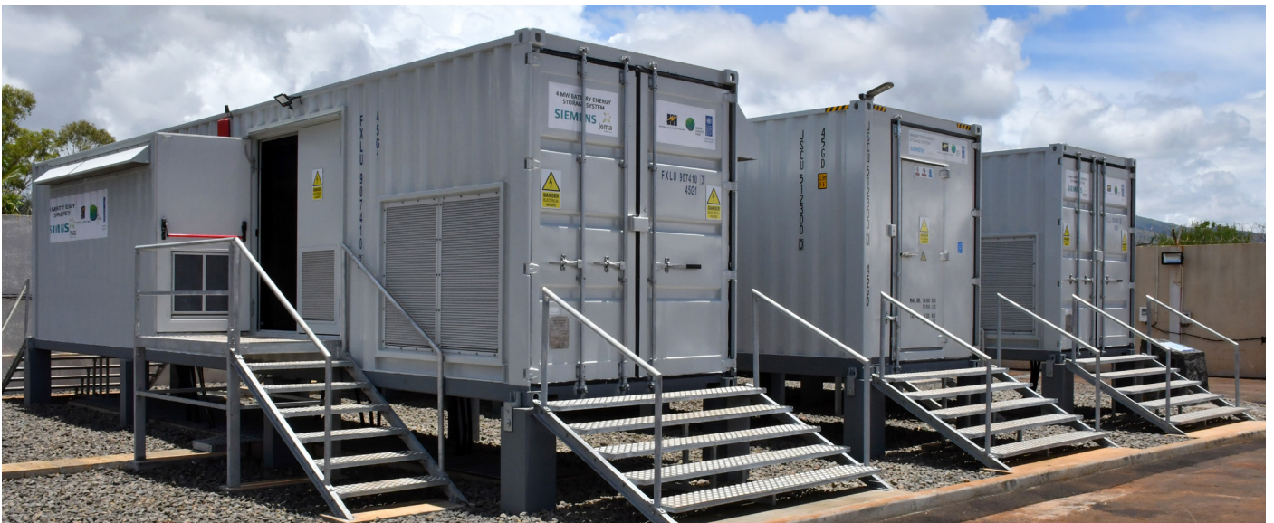
20MW Battery Energy Storage System (BESS) - CEB
