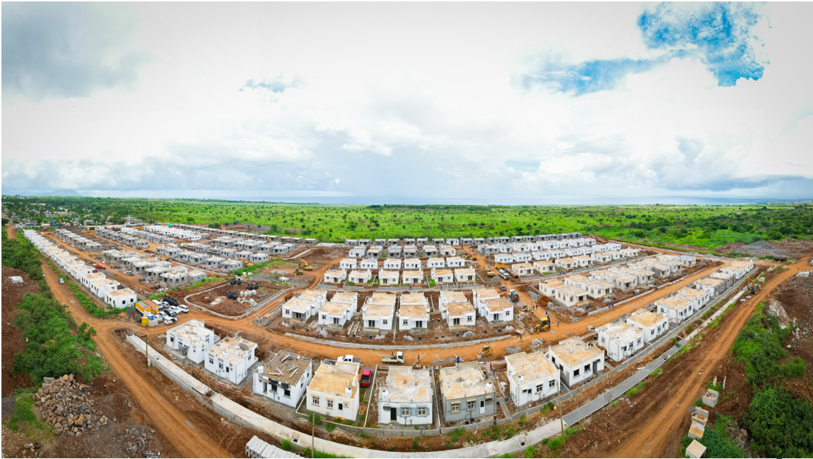
Construction of 108 Housing Units, Community Centre and Associated Infrastructure Works at La Valette 2, Bambous - NHDC
