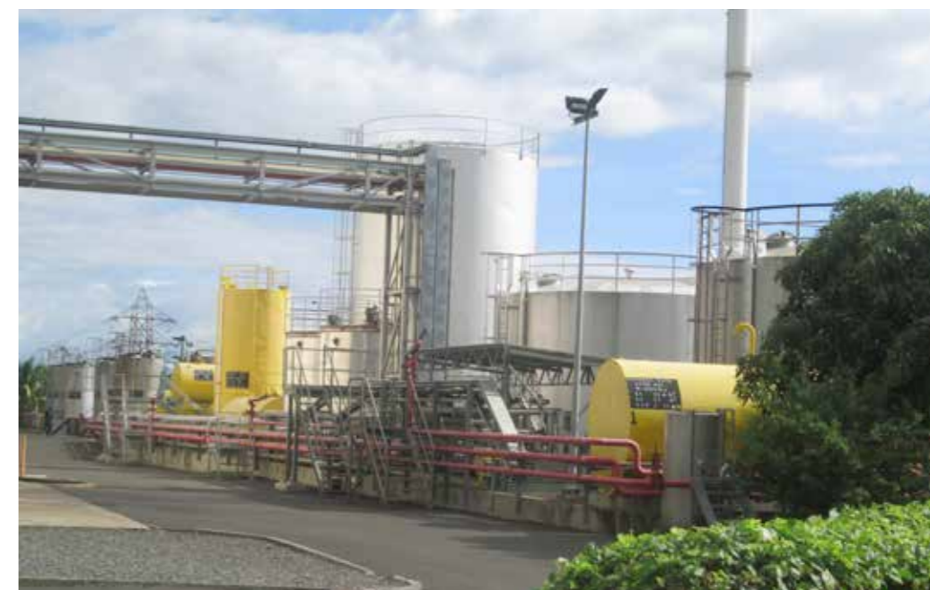
Figure 26: Supply of Lubricating Oil at St. Louis Power Station
