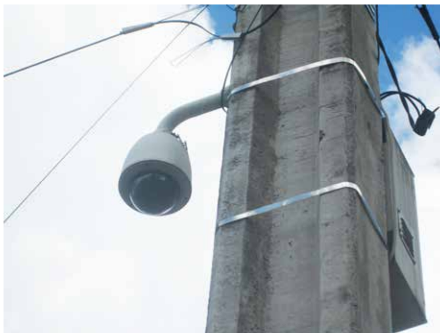
Figure 20: CCTV Camera in Quatre-Bornes
