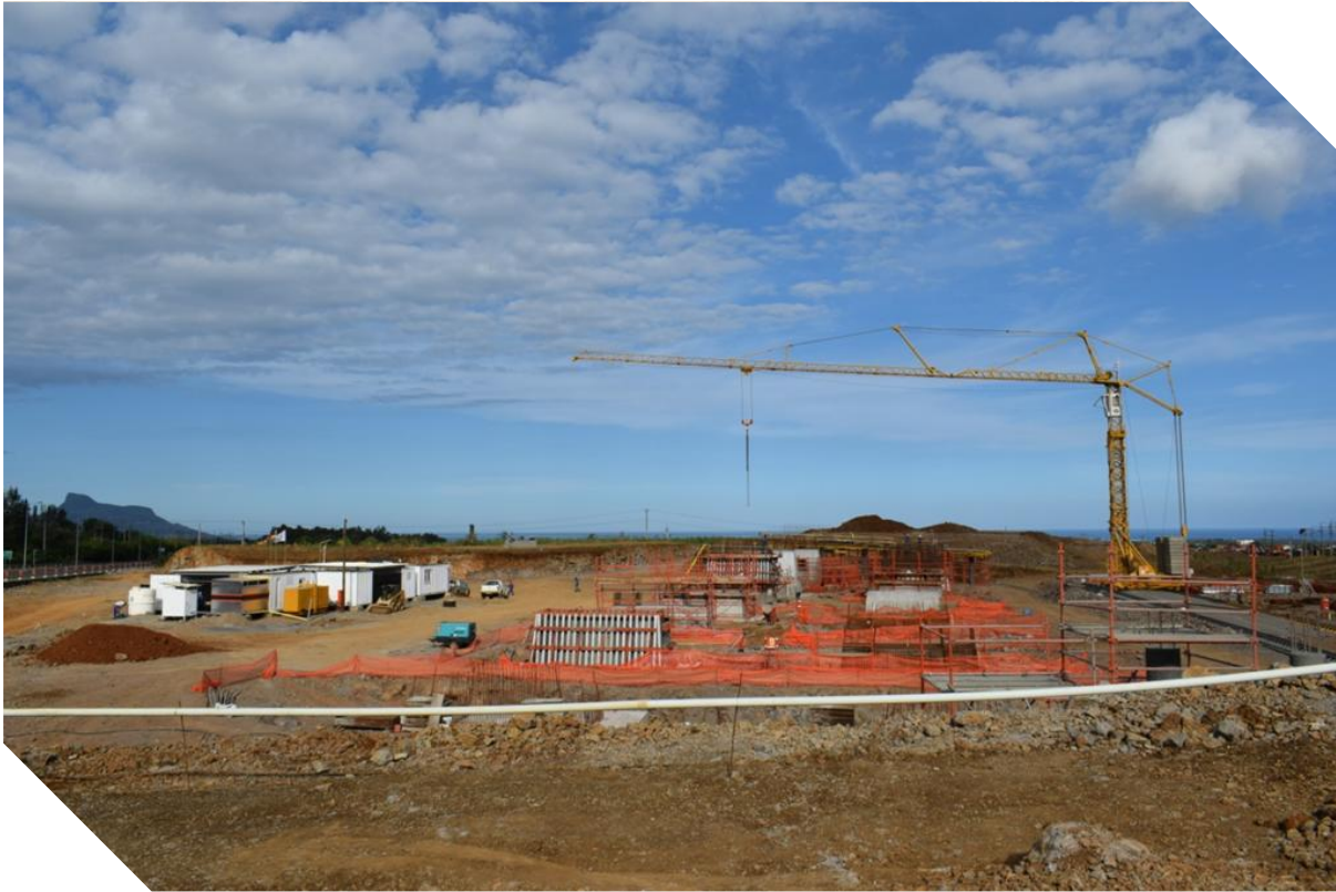
Construction of a New Airport Access Road to SSR International Airport - RDA
