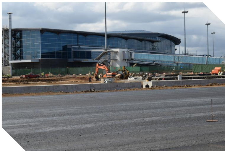
Aircraft parking stand No. 16 and installation of passenger boarding bridge on stand No. 15 – AML
