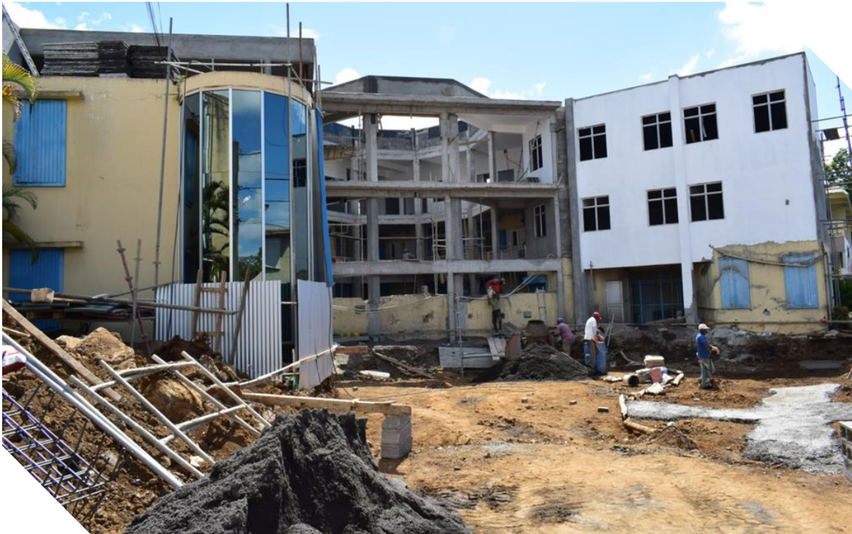
Construction of New Administrative Block and Extension Works to Existing Building at the Conservatoire National de Musique François Mitterrand
